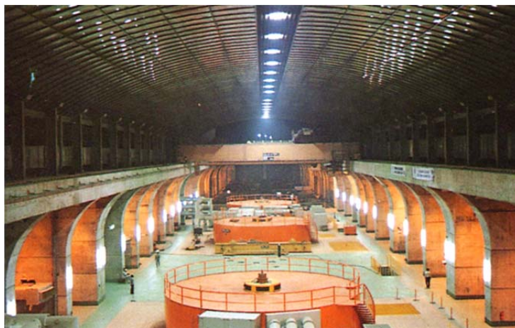
Underground Powerhouse, 25 m wide, 49.5 m high and 253 m long, capable of housing additional 500MW turbine-generators
