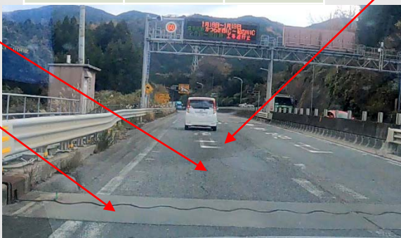
Photograph of the condition of the road surface
