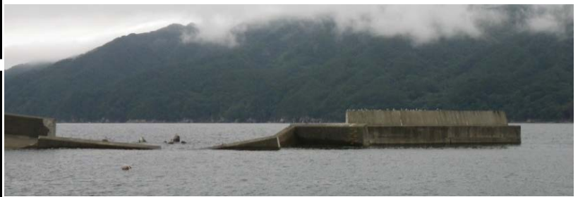
Example of damage to a breakwater (reconnaissance survey of Miyako/Kuji)
